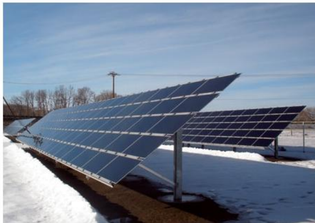
Innovative financial models such as virtual net metering can maximise solar potential (Source: University Park Solar)
